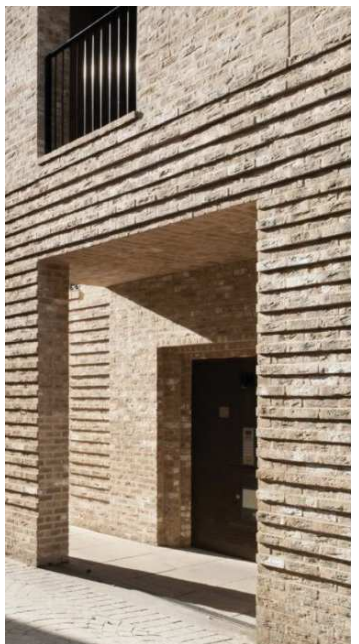
Example of brick feature at ground floor level for Blocks AB & CD
